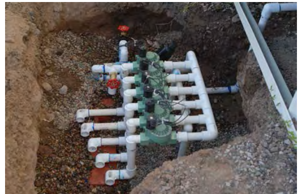
Drip irrigation valve manifold
